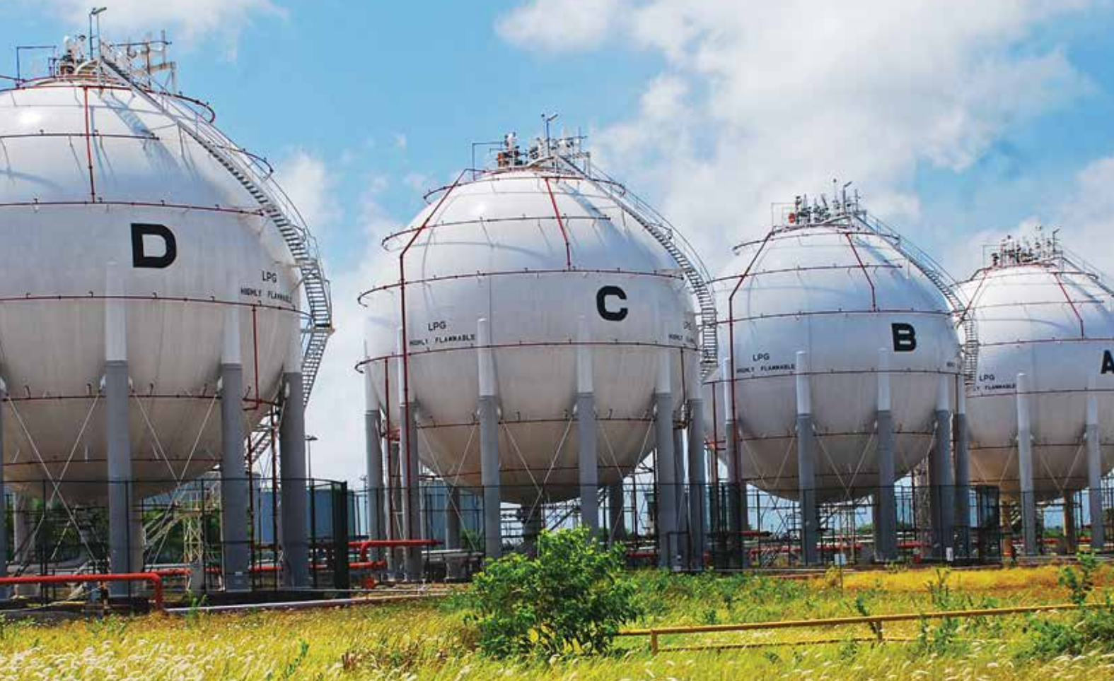
LPG Storage Tanks for Shell Terminal Lanka
