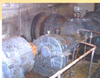
Condition of machinery & equipment before repairs
